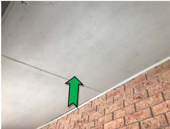
Photo 3. Exterior, ground level, south-east elevation, eaves – assumed non asbestos-containing fibre cement sheeting.
