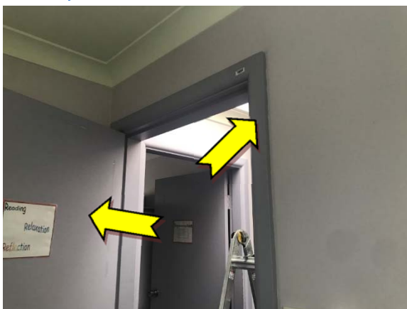
Photo 17. Interior, level 1, throughout, doors, window & door frames – suspected lead-containing dark purple upper paint system.
