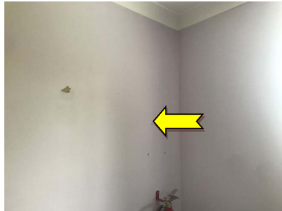
Photo 16. Interior, level 1, throughout, walls – suspected lead-containing purple upper paint system.
