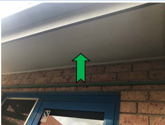
Photo 5. Exterior, ground level, south-west elevation, eaves – assumed non asbestos-containing fibre cement sheeting.
