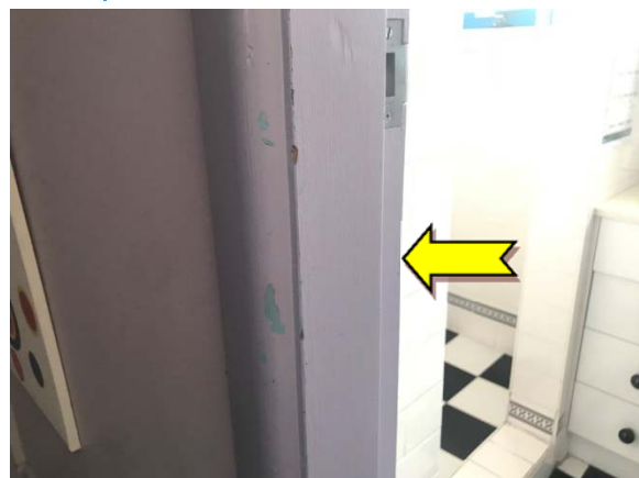
Photo 18. Interior, level 1, throughout, door frames – suspected lead-containing blue lower paint system.
