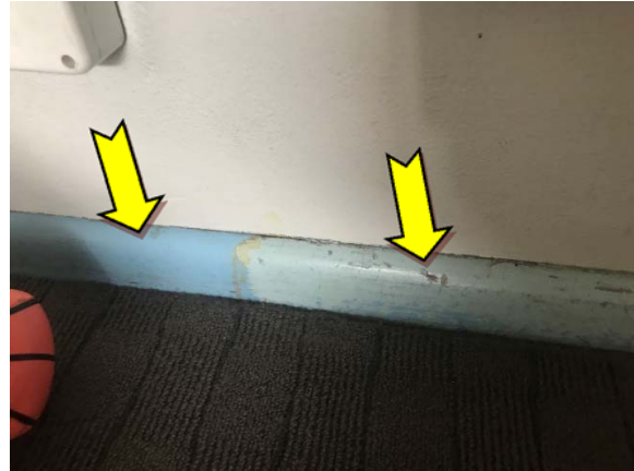
Photo 20. Interior, ground level, throughout skirting board – suspected lead-containing light blue lower paint system & dark blue upper paint system.
