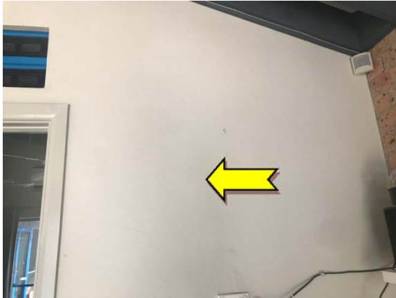
Photo 19. Interior, ground level, throughout, walls – suspected lead-containing light green paint system.
