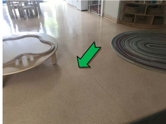
Photo 8. Interior, ground level, playroom, brown floor coverings – suspected non asbestos-containing sheet vinyl.
