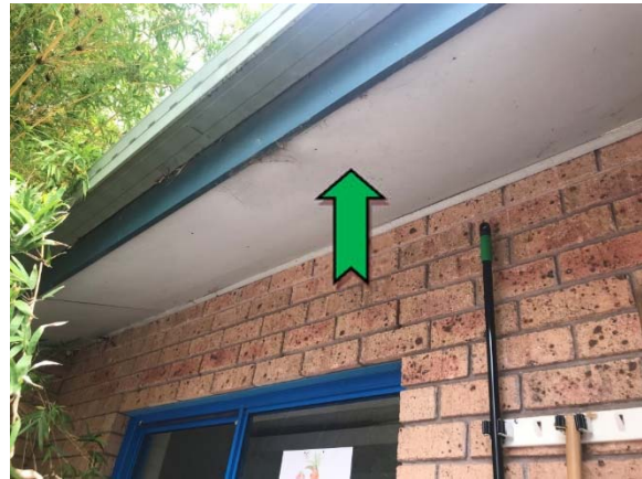
Photo 4. Exterior, ground level, south elevation, eaves – assumed non asbestos-containing fibre cement sheeting.
